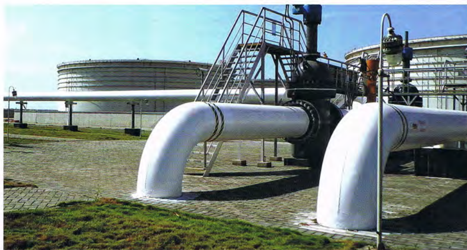
Carbon steel pipe used in gathering, processing, transportation or storage can use ceramic coatings.
