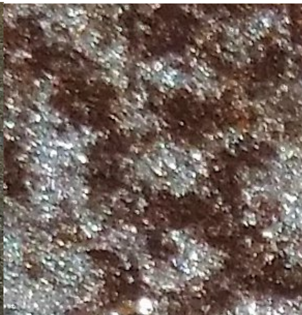
NOT ACCEPTABLE - Fe 2 O 3
