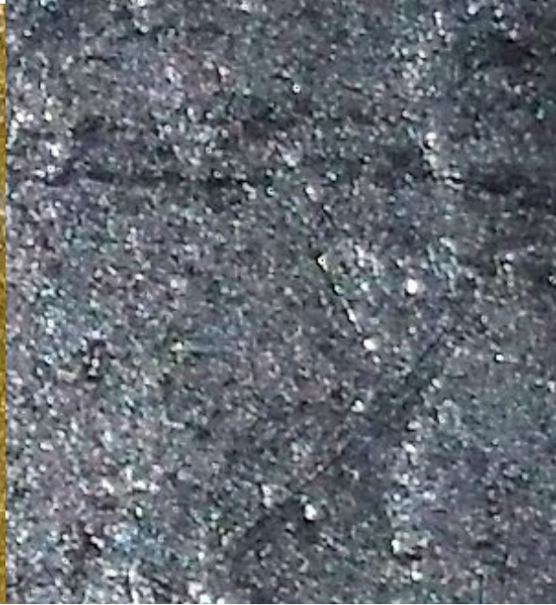
NOT ACCEPTABLE - MILL SCALE
