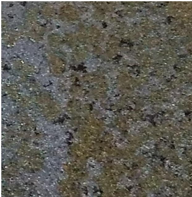
ACCEPTABLE - FLASH RUST & MINOR STAIN
