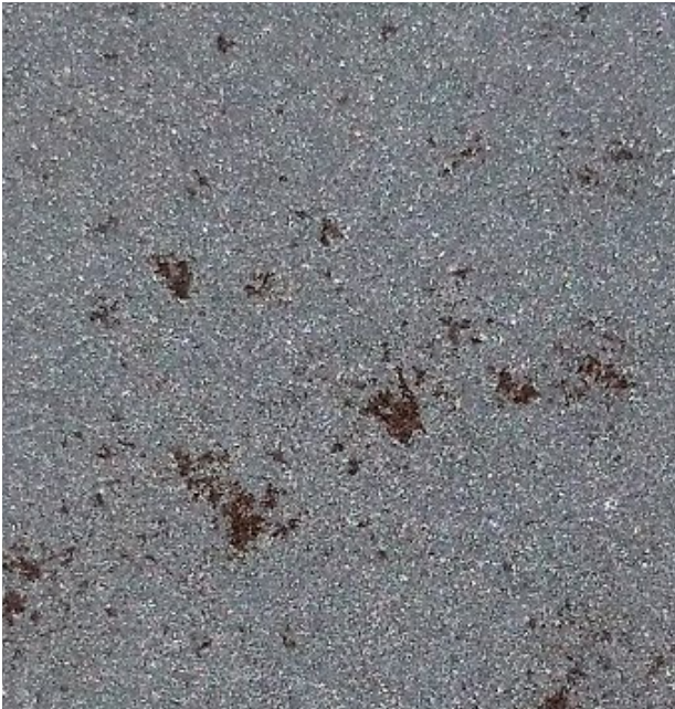
ACCEPTABLE - MINOR STAINING
