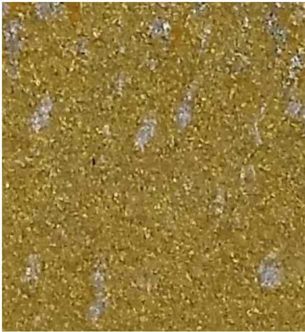
ACCEPTABLE - FLASH RUST
